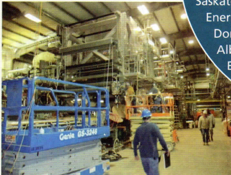
Burrows Paper has completed work on the extensive rebuild of its PM 41 at Pickens, MS. Metso supplied a new 15-ft MG cylinder and integrated hood. A new winder was also installed.
